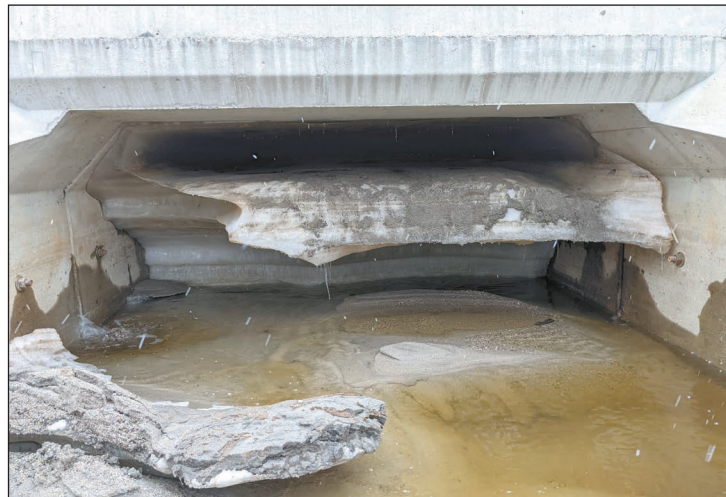
A SOLID BLOCK OF ICE formed in each of two 9-by-5 foot culverts in Poppleton Township, northeast of Lancaster recently. As shown above, no water is flowing through due to the solid wall of ice. (Submitted photo)
