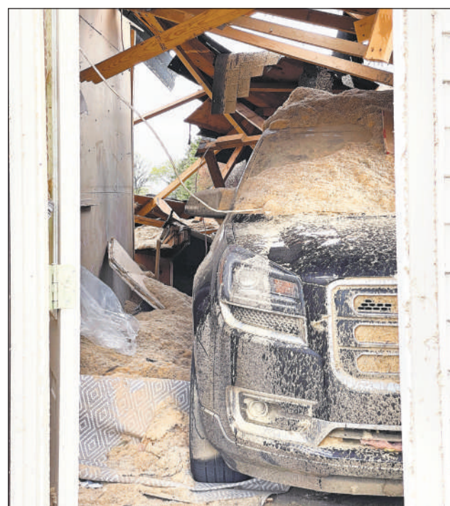
A vehicle covered in debris sits under a collapsed roof at the home of Dustin and Desiree Wiita of Alexandria. The family lost not only their home, but both vehicles that were parked in the garage after a tornado ripped through their neighborhood along South Darling Drive on May 12.
