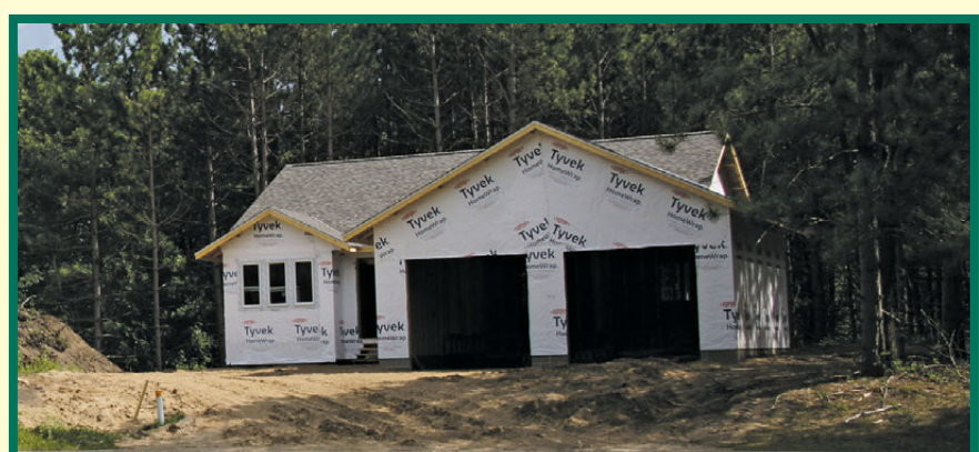
Now Under Construction on Lot 36 This home is on the largest of these 10 lots and features stainless steel appliances, a main-level laundry, and a walk-out, ready-to-finish basement.
