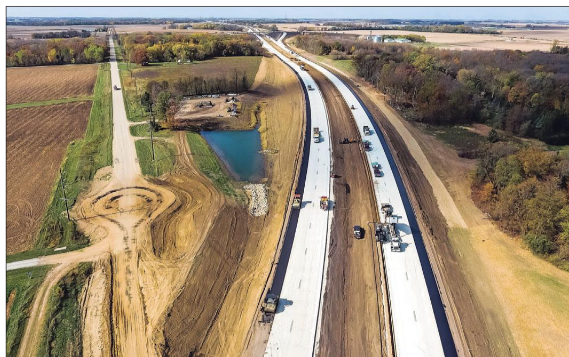
The new Highway 14 cuts through farm fields near Dodge Center. Photo taken Oct. 19.
