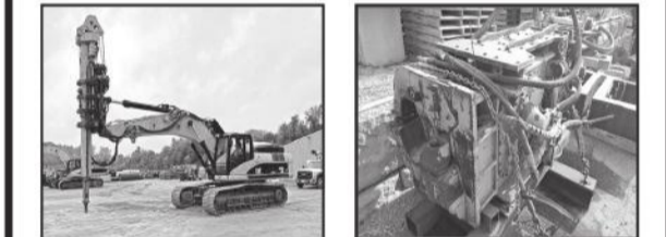
D11111 '07 CAT 330DL excavator w/ Bay Shore Systems LoDril KK9148 Movax SP-100 excavator vibratory pile driver
