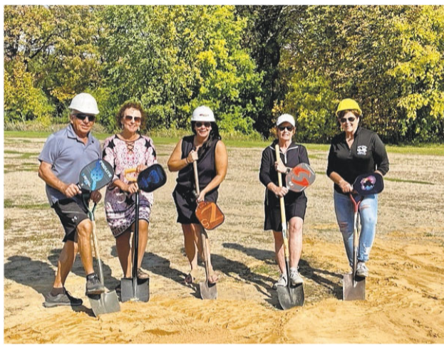
Left: Vergas Pickleball Court Committee members, from left, Ron Franklin, Sherri Hanson, Maria Sontag, Shannon Charpentier and Jill Shipman, dug into the ground for a groundbreaking ceremony before bulldozers arrived earlier this fall. Right: Bulldozing on the Vergas pickleball courts started Oct. 16.
