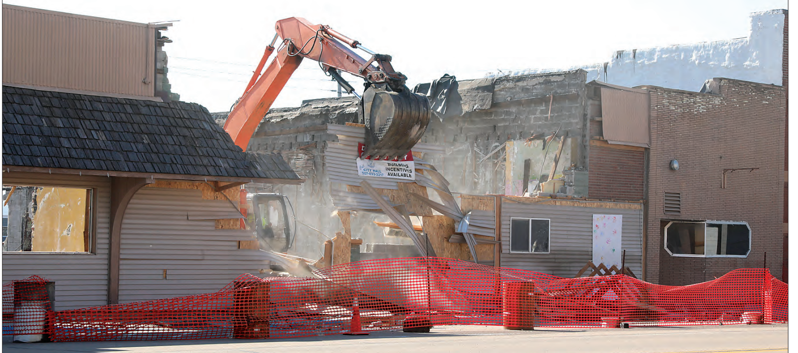
The long-anticipated demolition of Winnebago's SuperValu building on Main Street finally began on Monday, June 27. The process took several days. Demolition started at the back of the building before the construction crew made it to the Main Street-facing store front. A crane gouged through the front of the building mid-week, as pictured above.
