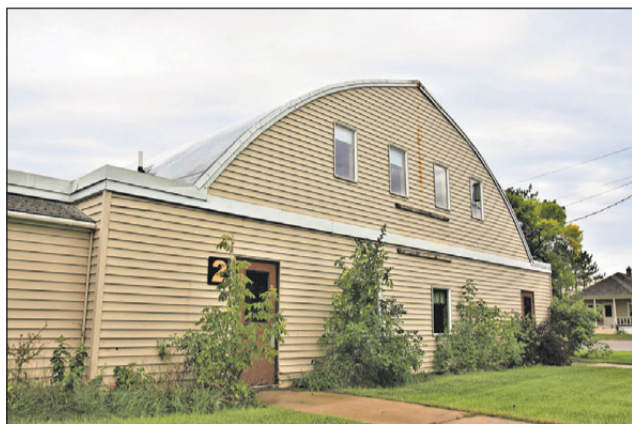
Elizabeth Vierkant / Perham Focus Construction has started on the old 4-H building to make it suitable for Productive Alternatives.
