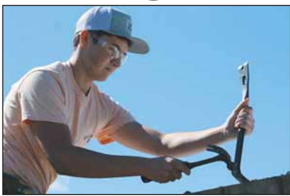
A pry bar and a hammer were used to pull up nails or screws attaching the tin to the roof of the dugouts.
