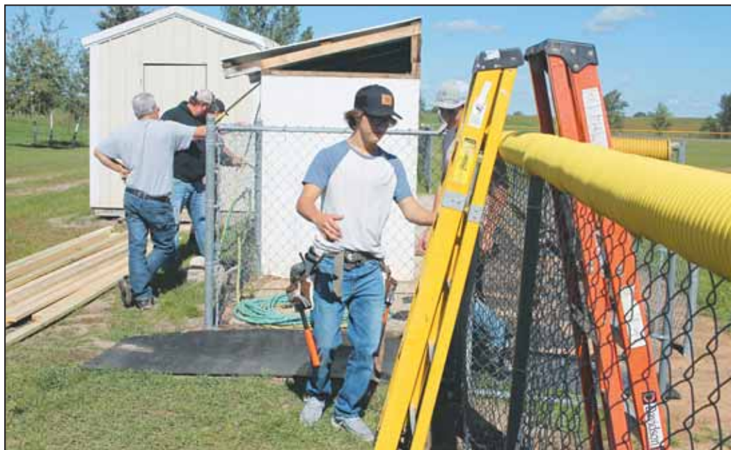
Students in the construction trades class grabbed ladders to begin removing the tin roof on the baseball dugout. Photos by Barbie Porter
