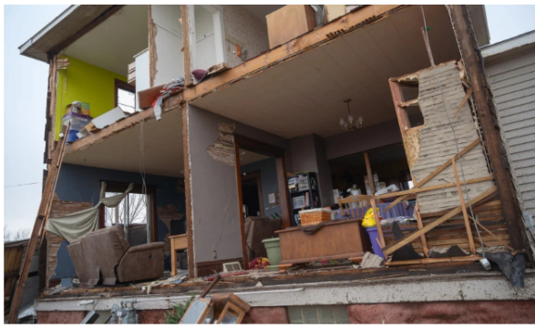
The wall of a home is missing on Wednesday, April 13, 2022, after a tornado the night before in Taopi, Minnesota. The National Weather Service confirmed an EF2 tornado touched down in Taopi. Joe Ahlquist / Post Bulletin
