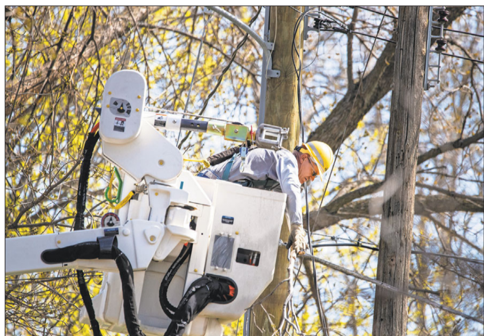
John Zvorak of Otter Tail Power Company removes branches from power lines Friday morning in Murdock.
