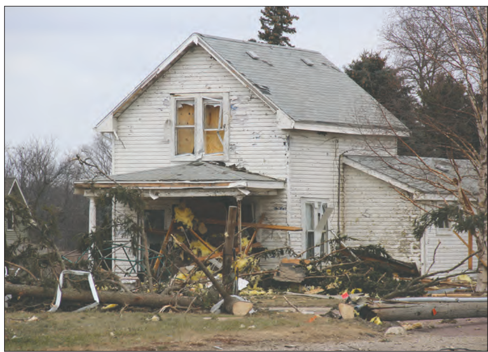
A house owned by J.R. and Joyce Henderson sustained severe damage in Hartland from downed limbs and debris from nearby homes.
