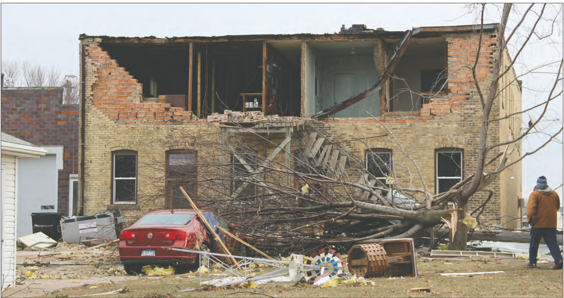
The back wall of the building in downtown Hartland that hosts the post office was ripped off Wednesday night during severe weather. Several buildings along Broadway and houses in the immediate area were damaged from what the National Weather Service has confirmed was an EF2 tornado. SARAH STULTZ/ALBERT LEA TRIBUNE
