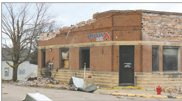
Arcadian Bank in Hartland sustained severe exterior damage Wednesday night during a storm that came through the area.
