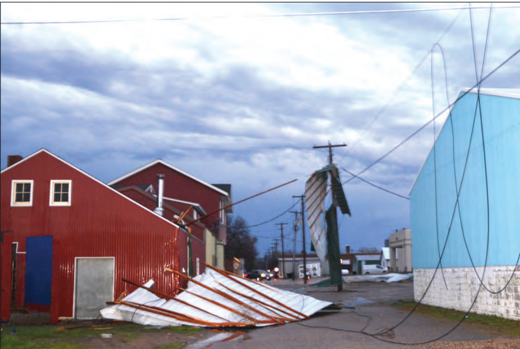
A mass of downed power lines and pieces of the Glacial Plains Cooperative feed shed roof littered the business alley in Kerkhoven between Windy's Wellness and the Butcher Block building. Otter Tail Power crew members worked through the weekend to restore power to homes and businesses.
