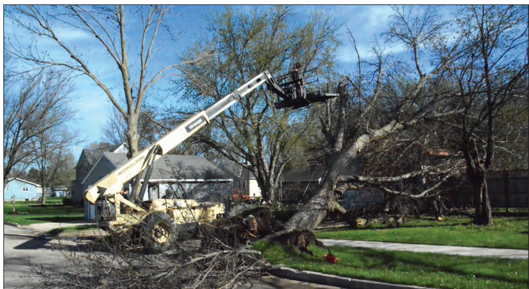
A worker used a boom to cut away branches from a large tree which blew over onto the garage at the Lucas and Katelyn Friedlein yard in Kerkhoven.
