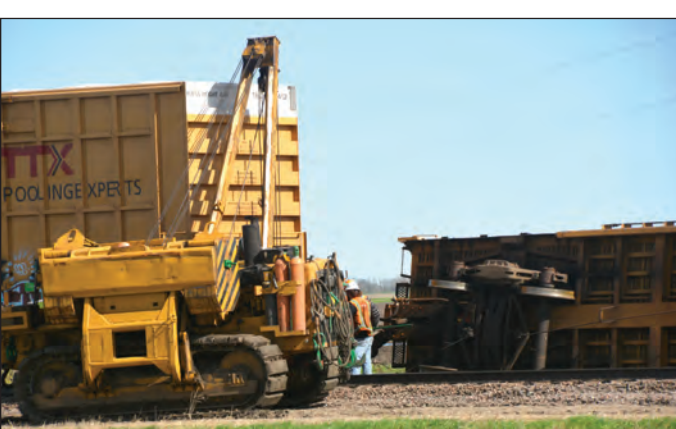
Heavy equipment was brought in to right several rail cars which were blown off the tracks by Pennock.
