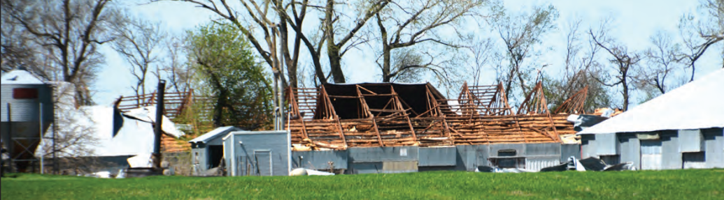
A turkey barn near Murdock lost its roof in the storm, blowing metal and insulation across Highway 12 and into a farm field.
