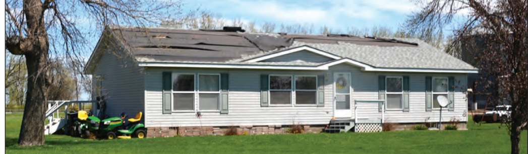
This DeGraff house had lost much of its shingles in the brief but powerful Thursday night storm. Roof damage from wind or falling trees was abundant.
