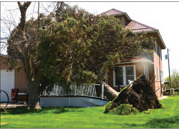
A large tree crashed into the front porch of this DeGraff house.
