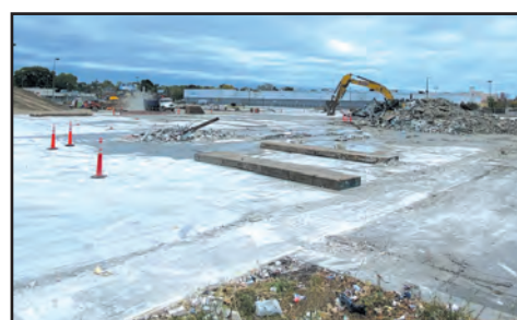
A backhoe eats through the remaining rubble at the Midway Center on Oct. 12, 2021. (Photo by Tesha M. Christensen)
