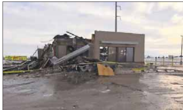
Photo courtesy of Nathan Peterson The Jackson Burger King is shown following a fire that began late Friday night and required the services of six regional fire departments.
