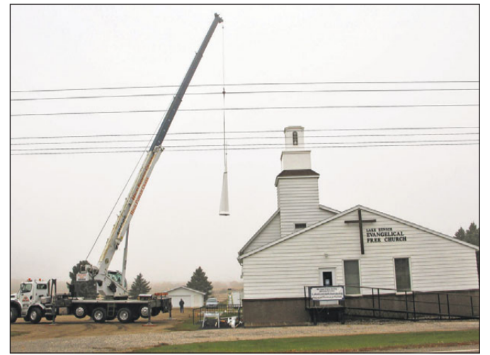
The final piece of a new 35-foot church steeple, the spire, is hoisted into position for installation.
