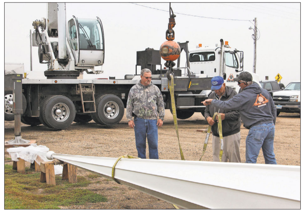
Volunteers prepare to hoist the spire of the new 35-foot church steeple.
