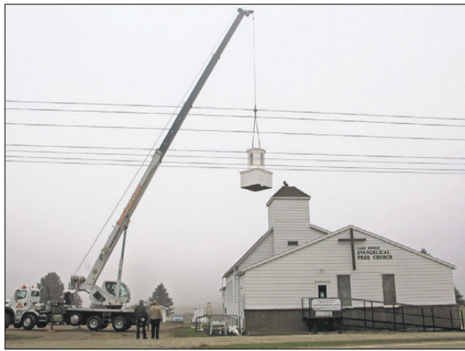
The two-part base of a new 35-foot church steeple is hoisted onto an existing church tower.
