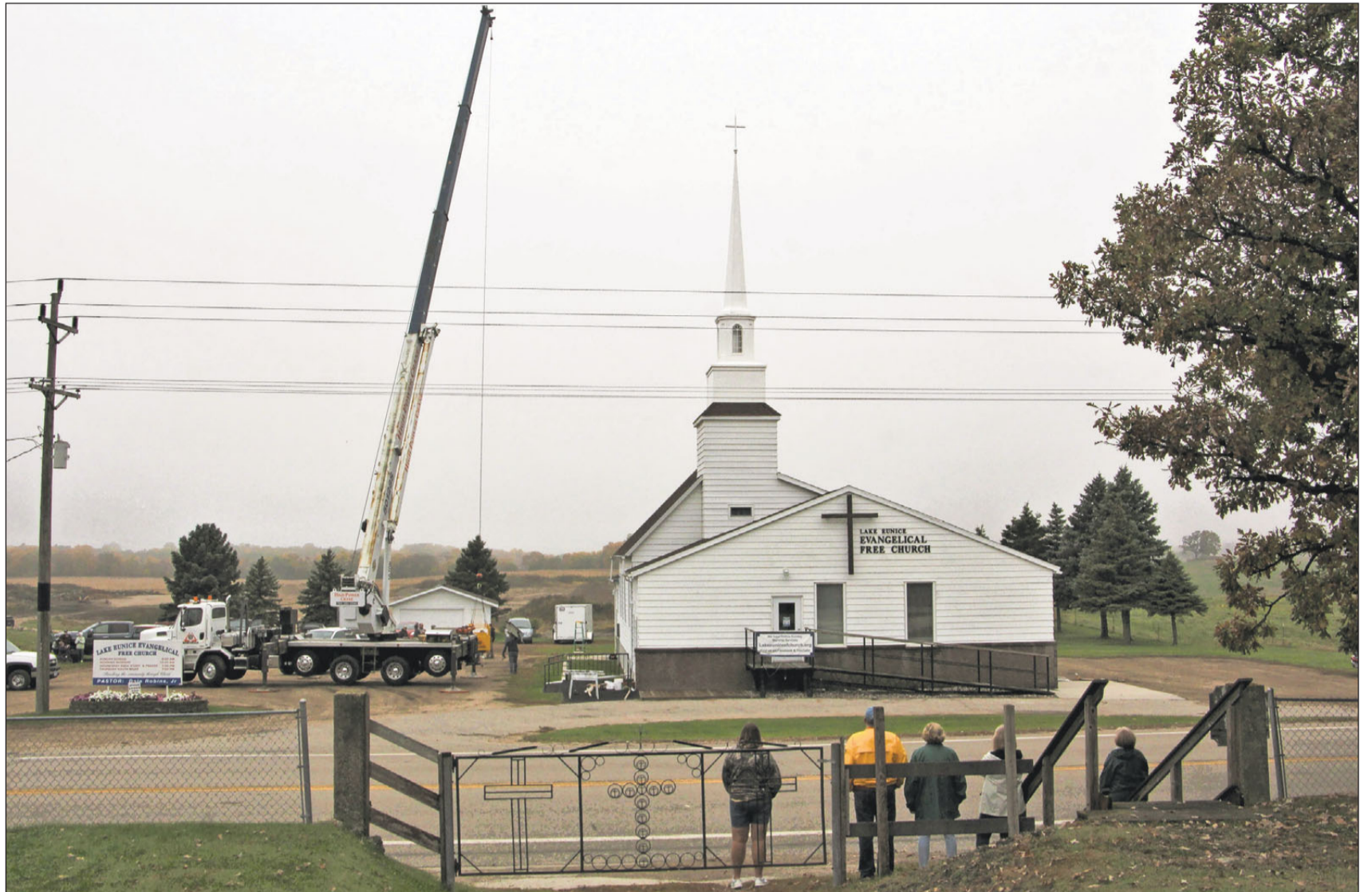
Onlookers view the completed installation of Lake Eunice Evangelical Free Church’s new 35-foot steeple. The church received the steeple as a gift from a hometown parishioner.
