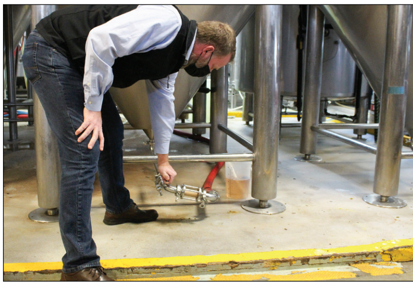
Lift Bridge CEO Dan Schwarz opens the valve on Wednesday, Dec. 16, to empty out a beer distiller to make room for beer the craft brewery is brewing. (Gazette staff photo by Matt DeBow)
