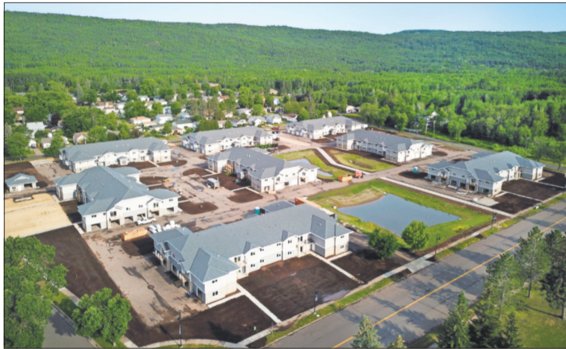
The Morgan Park Estates development on Thursday, June 24, 2021. Eight 12-plex buildings are being finished on the former site of Morgan Park School.
