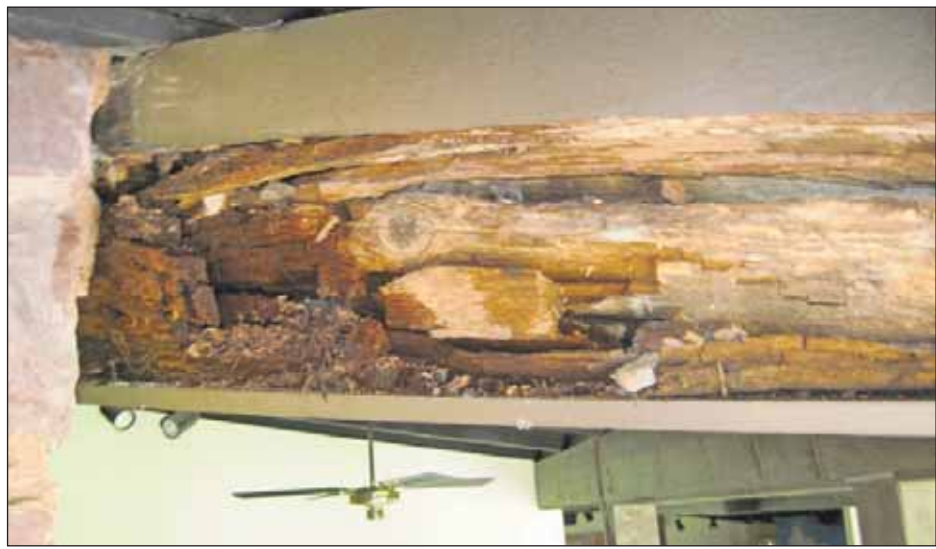
A load-bearing beam inside the Blue Mounds State Park Interpretive Center shows significant rot in this image. The rot was discovered in 2015, leading to the center's closure.
