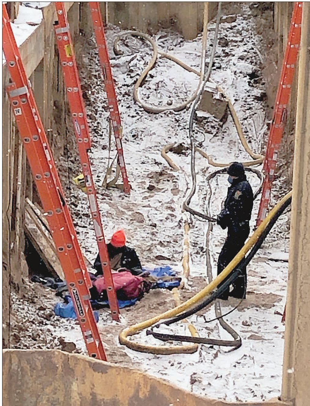
A tribal police officer stands near protester Phoenix as she reads in a pit created for pipeline construction off Reponen Road west of Cloquet. The woman was arrested a short time later. Photos courtesy Rachel Sipress
