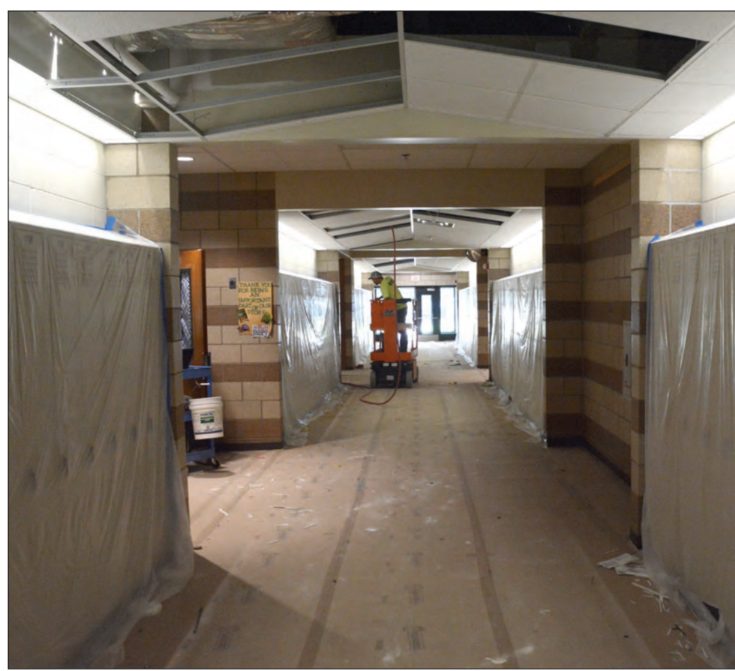
Walking in the hallways of KMS High School this week, it doesn't look like school is just days away from starting a new term. Contractors have been replacing worn HVAC lines and units for
