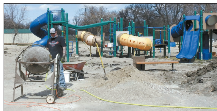
HALLOCK CITY MAINTENANCE EMPLOYEES worked on completing the equipment installation at Gilbert Olson Park last week. Here, Caleb Pinnock mixes cement to finish up installing support poles while Joel Peterson and Utilities Superintendent Dan Larson work on the other side of the equipment. Once the equipment is completely installed, the crew will clean up the loose, ripped landscaping fabric, lay down new fabric and replace the pea rock. They hope to have this project complete by Memorial Day weekend. (Enterprise photo by Anna Jauhola)
