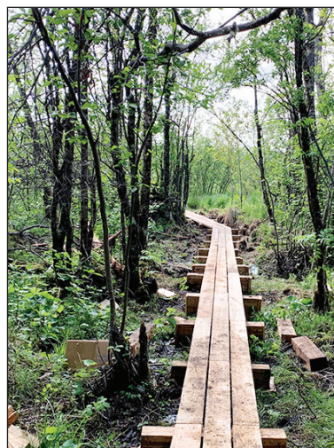
Left: The new boardwalk makes its way through a wetland as the first leg of the new Ancient Cedar Forest Trail now under construction in Tower.
