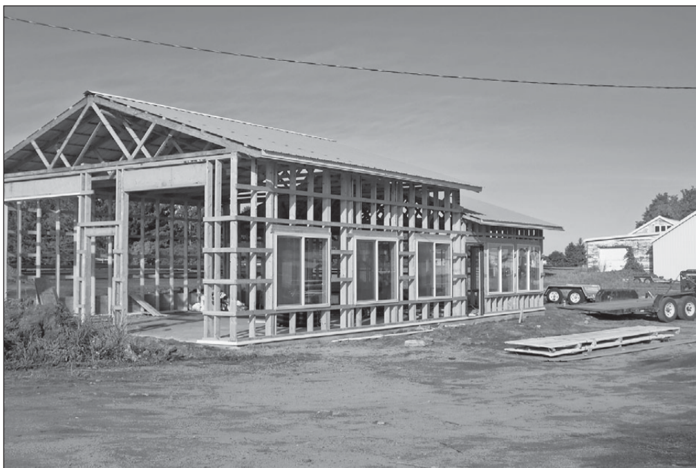
At the corner of SW Second St. and Hwy 10, a new Lunde Auto Sales shop and sale lot is being constructed. They originally planned to use the former Carter Oil building but the foundation was not usable.
