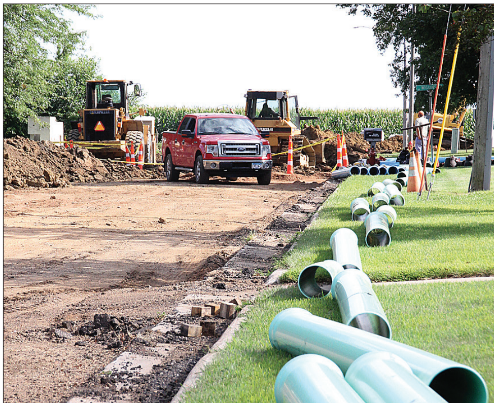
STORM SEWER WORK WALNUT GROVE — Last Tuesday afternoon this crew was busy installing a new sanitary-sewer at the east end of Wiggins Street on the southeast part of Walnut Grove. (Photo/Tom Merchant)
