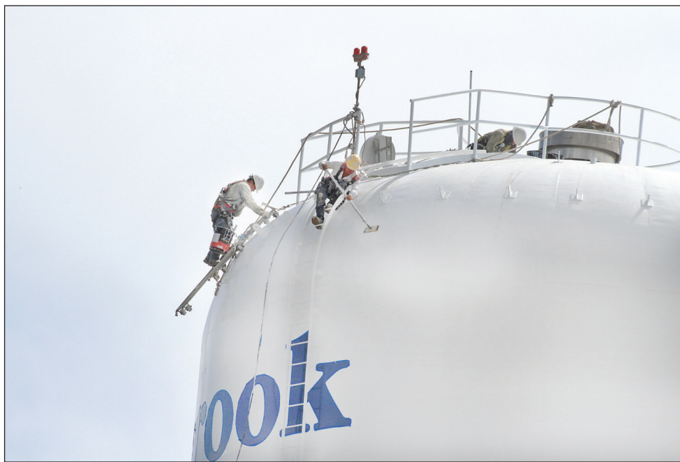
PUTTING ON THE FINISHING TOUCHES WESTBROOK — Last Thursday morning this water tower paint crew were busy adding finishing touches to the water tower painting project. (Photo/Tom Merchant)
