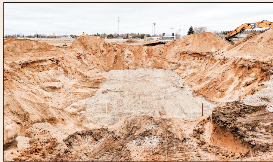
Matt Uselman snapped a picture of the work that has been done at the new well site near Verndale Custom Builders on Highway 10. Below, a crew installed a billboard at the gas station on Highway 10.
