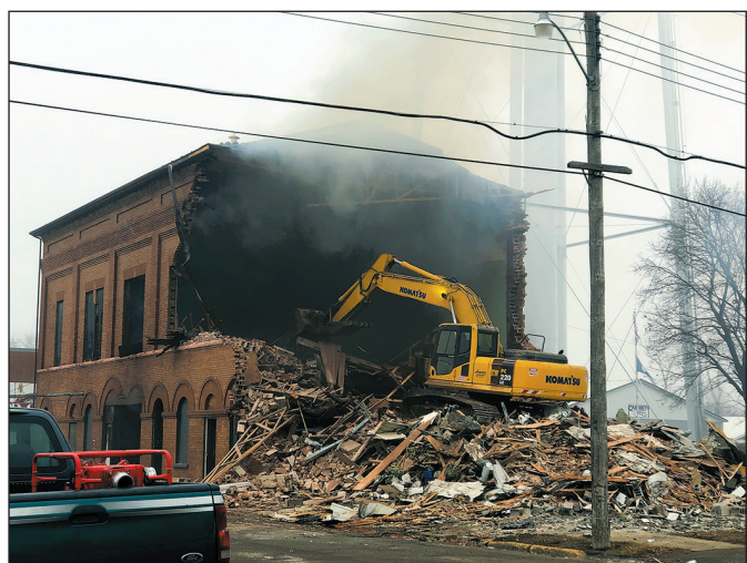
Alyssa Sobotka / The Globe Demolition is shown Tuesday morning at Ellsworth's City Hall following a fire that rendered the building a total loss.
